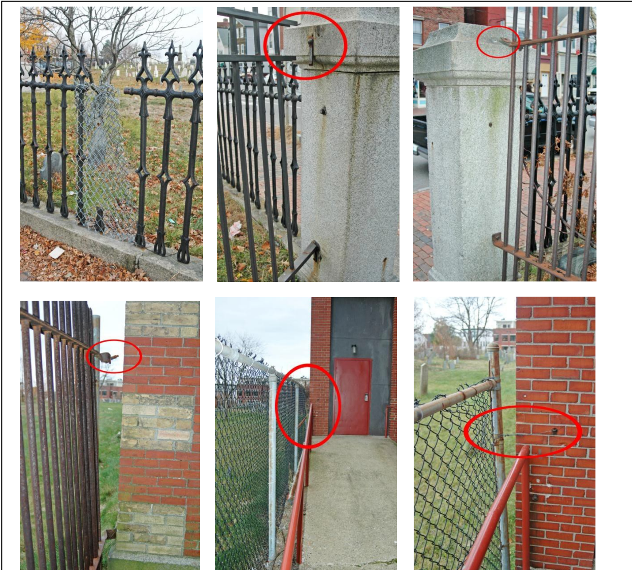
Figure 55. Fence problems that require immediate action. Upper left shows damaged section on Congress Street that allows ready access to the cemetery. Upper middle shows the damage to the connector at the corner of Congress and Mountfort streets. Upper right shows the damaged connector on Congress at the North School line. Lower left shows the damaged connector attaching the fence to North School. Lower middle shows that the fence along the North School ramp is not high enough to prevent entry. Lower right shows the damaged connector of the chain link fence to North School. Not shown is the damaged fence at the south edge of the cemetery along the rooftop of adjacent businesses.
