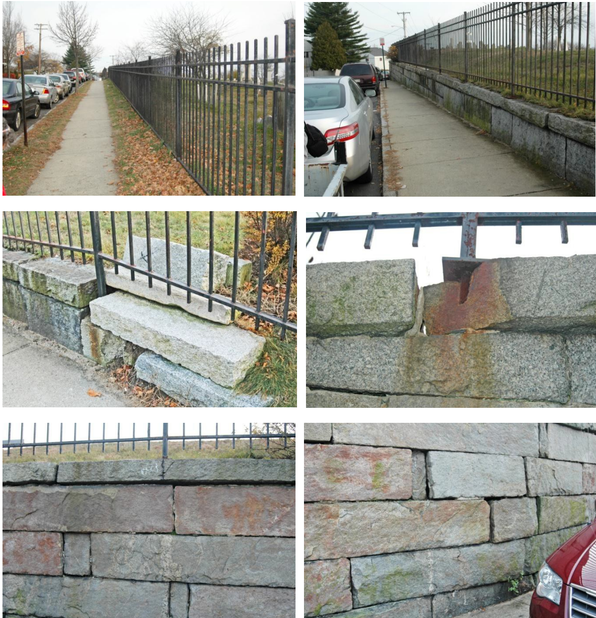
Figure 58. Mountfort Street fence and wall. Upper left photo shows the fence, looking to the northeast. Upper right shows the fence set on the granite retaining wall. Middle left shows where the granite wall has been “extended” by dumping granite coping. Middle right photo shows where iron jacking has split the granite coping. Lower left photo shows loss of mortar in the joints of the wall. Note also the crack that has formed from iron jacking at the line post in the center of the photo. Lower right shows a noticeable bulge in the wall on Mountfort. Joints are open and the retaining rock is set back in the wall, showing the movement outward.
