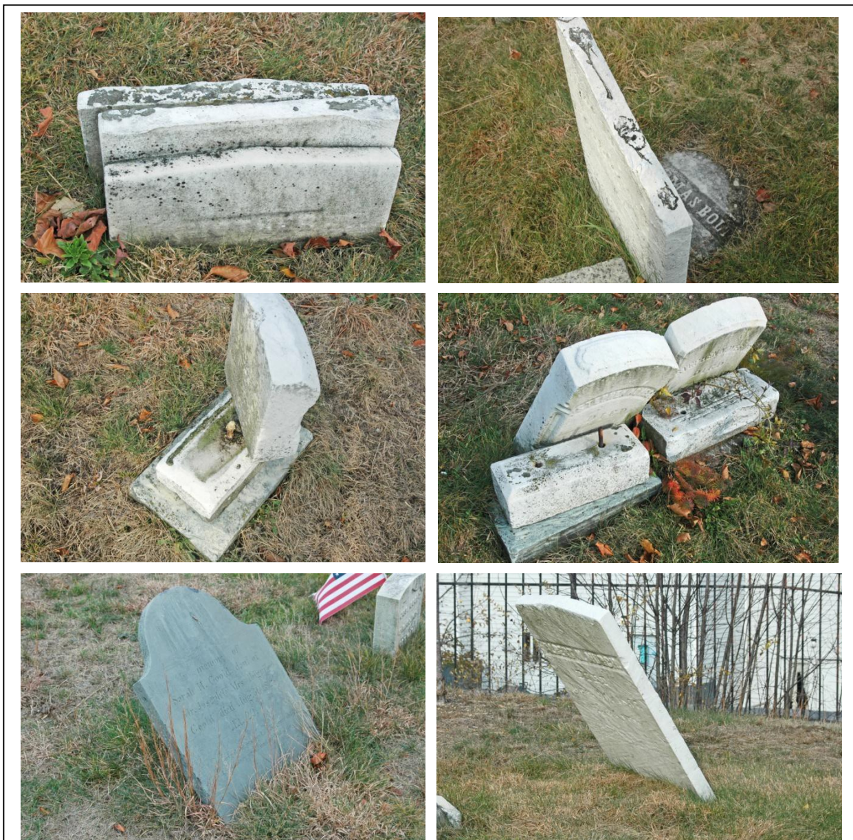
Figure 81. Conservation issues. Top row shows stones that have old “simple epoxy” repairs that have failed. On the left the stone fragments have been reset one behind another. On the right the top of the stone is still in the ground and subject to additional damage. These stones should be drilled and pinned, returning them to their original condition and promoting the three-dimensional appearance of the cemetery. The middle row show die on base stones with ferrous pins. The example on the left shows that the pin was set with brimstone, the old name for melted sulfur. Unfortunately sulfur promotes iron corrosion, exacerbating the likelihood of iron jacking. These should be removed and replaced with fiberglass pins. The bottom row of photographs shows stones with tilts in excess of 20°. Stones with such severe tilts pose a threat to themselves and should be reset as soon as possible.
